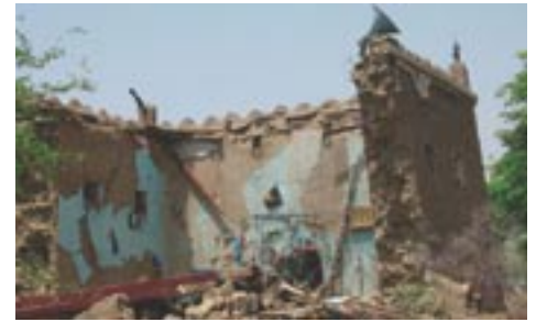
A Masjid damaged by floods in Pakistan
