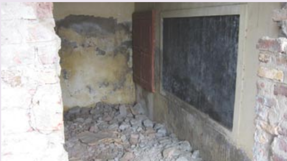
Classrooms have been looted and abandoned to the extent that even doorways have been taken
